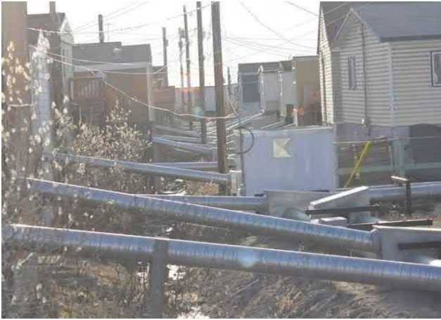
Figure 11: Inuvik's Water Treatment Facility (Credit: Mackenzie Scott/CBC)
